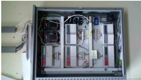
HVAC controls system used to reduce energy consumption during unoccupied hours.
